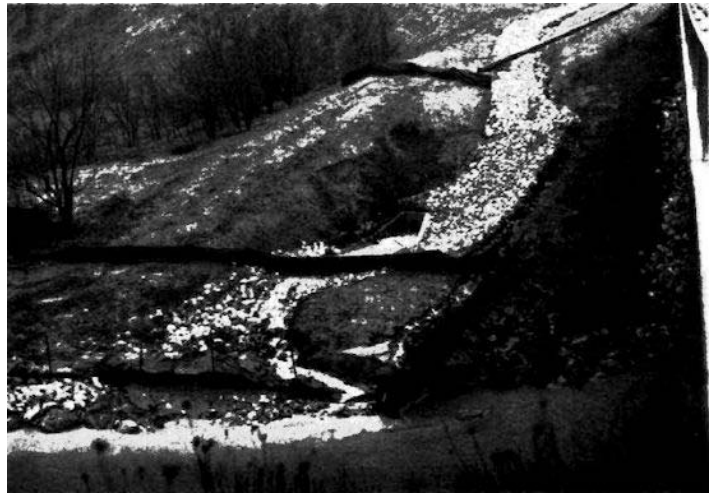
Fig. 1 Careless construction - Humber River.
