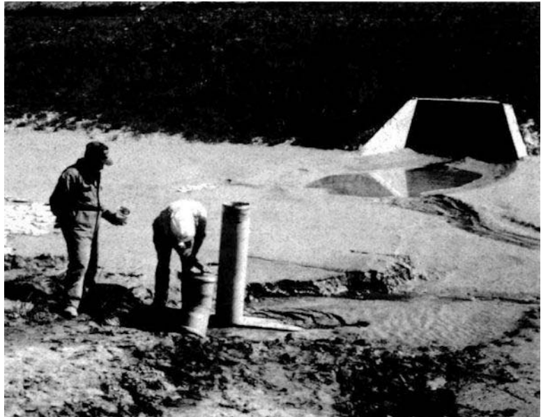
Fig. 11. Retrofit storm water management pond.
