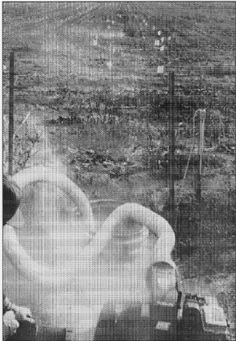
Figure 3 Smoke emitting from the ground following pressurization of the system.
