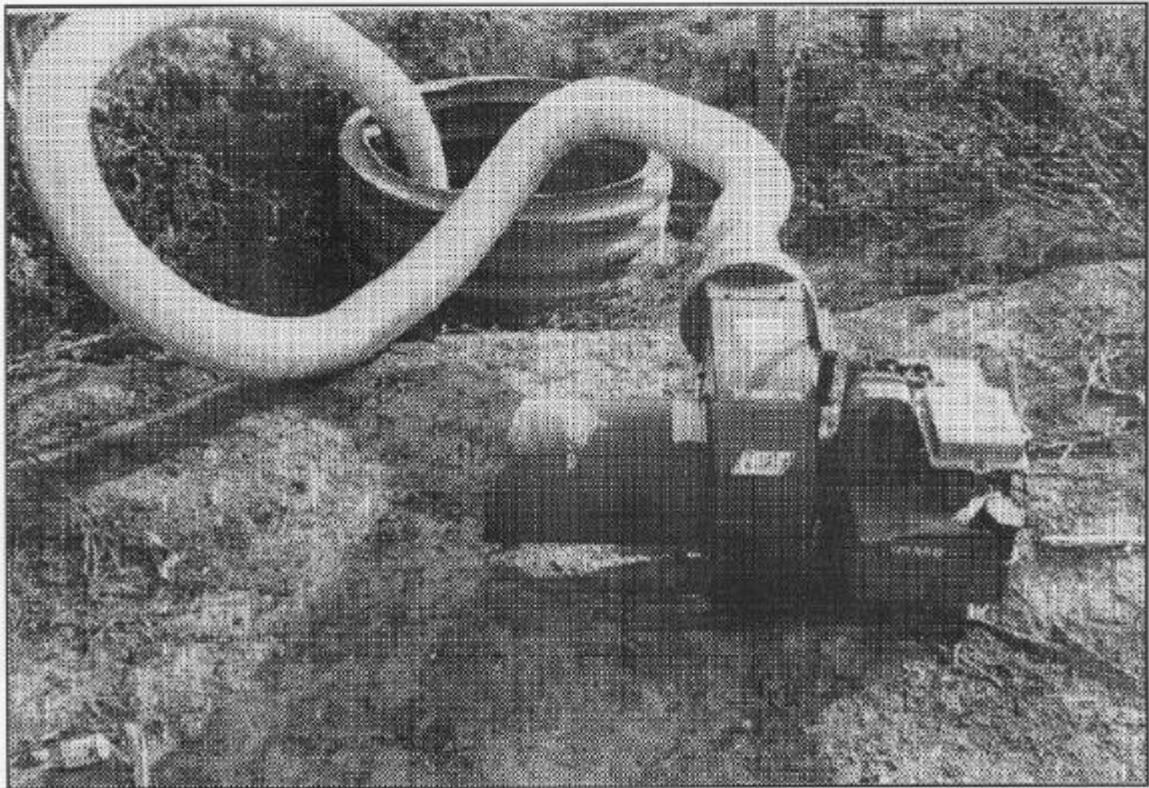
Figure 1 Typical setup of blower fan and pipe connecting to subsurface drain.
