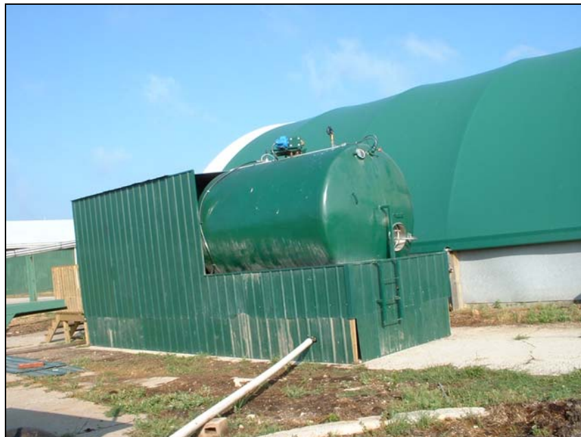
Figure 1 Pilot scale Anaerobic Digester #1 at the Ridgetown Campus – the mix tank is hidden and the main digester is the large tank on the right
